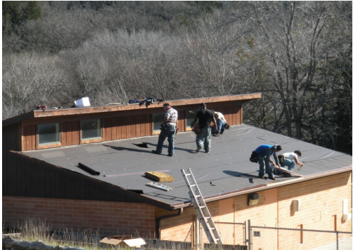
Following an insurance settlement for hail damage, several buildings at Moses Merrill each got a new roof. Crews took advantage of good weather in November to work on the project. This is the pool house.
