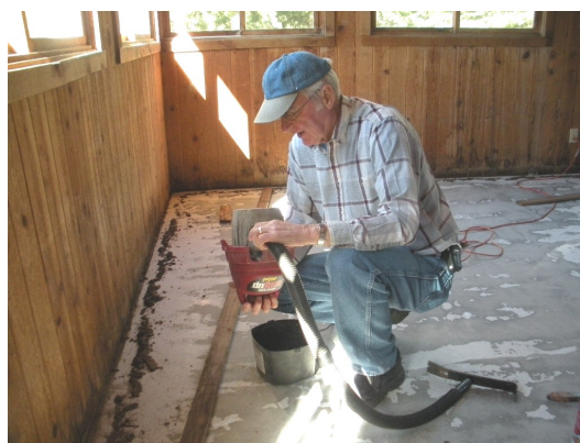
Paul Badje, FBC, Columbus, works on refinishing the floor of the Weaver Hall porch during Spring Work Week.
